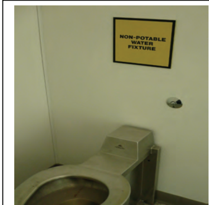
Harvested rainwater toilet flushing - Fort Bragg Community Emergency Services Building
